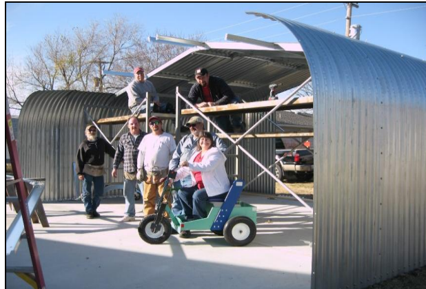
The straight sidewall and pitched roof design has the shape of a traditional gable. Here the work crew poses with Kirby and Chris (front right).
