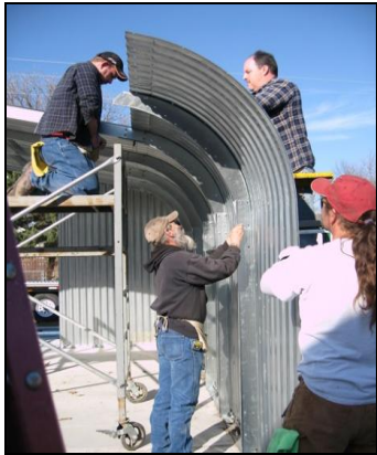
Workers assembled the outer structure of the arch on the new steel building.
